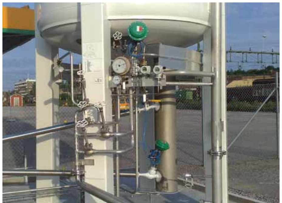
Sundsvall: HEROSE valves on the biogas tank
