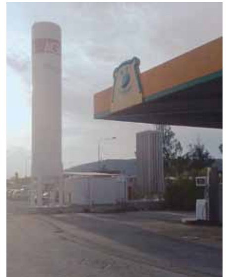
The biogas filling station in Sundsvall
