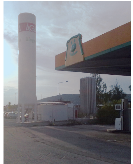
The biogas filling station in Sundsvall
