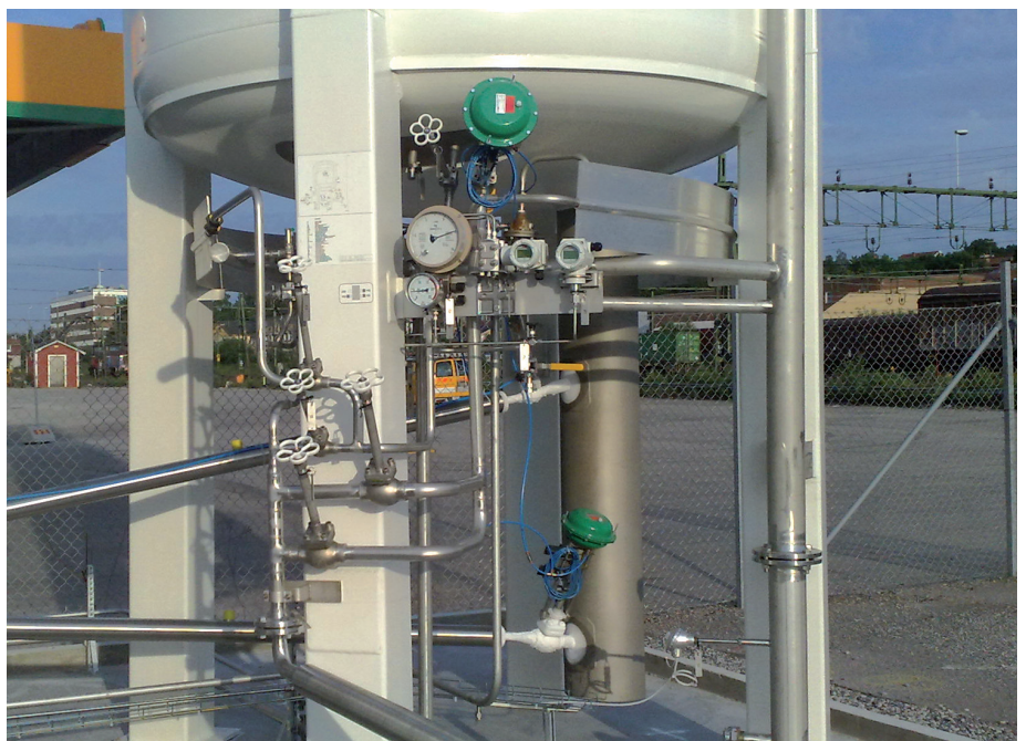
Sundsvall: HEROSE valves on the biogas tank
