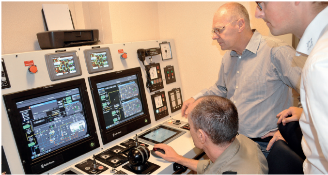
Chief Engineer Martin Walter explains the ship's LNG control system to HEROSE employees Mario Esche (right) and Manfred Kadner
