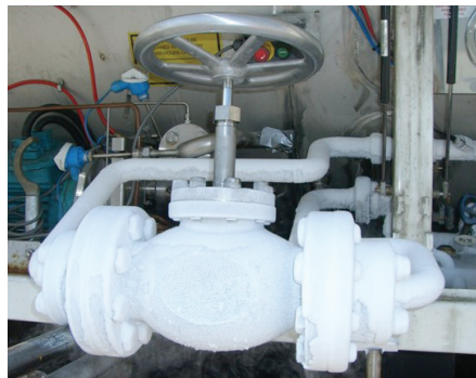
Cold shock testing as per DIN EN 12567 on an LNG trailer (tank truck)
